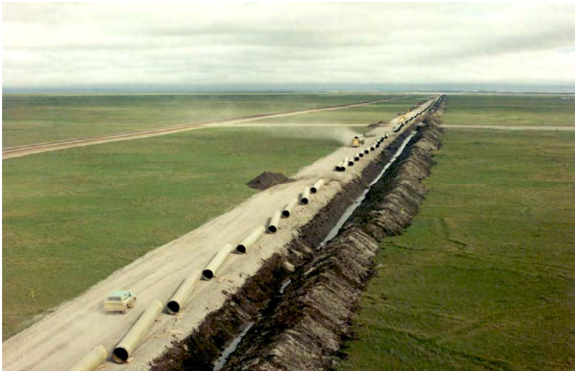
Figure 2. Pipelines are essential for transporting our oil and gas
