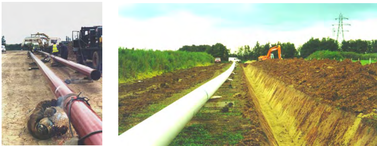
Figure 1. Most of today's oil and gas pipelines are welded together and buried underground or laid subsea
