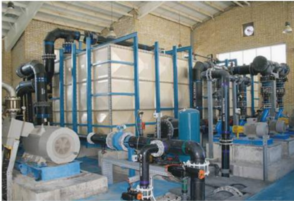
Chabahar–Kenarak RO desalination plant
