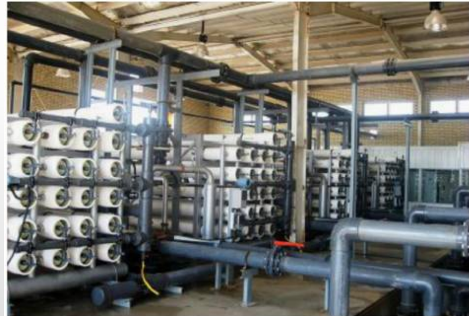
RO desalination plant installed in Bandar Lengeh
